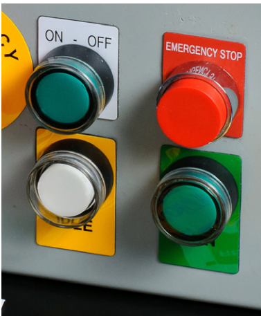
Control panel labels
