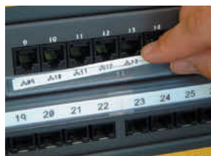
Punch block & patch panel labels
