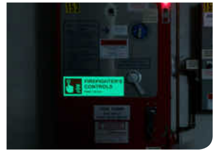
Exit & directional signs
